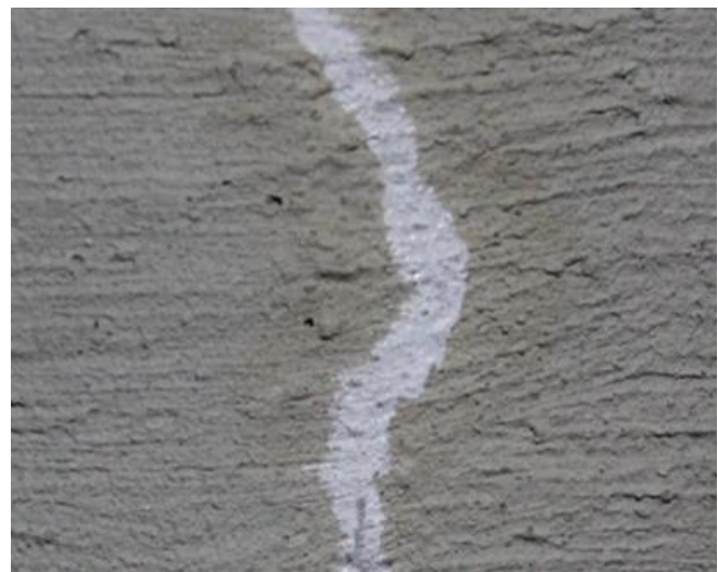
Photo 4. The crack is closed by salt crystals, no water seepage. Effect after 21 days.
