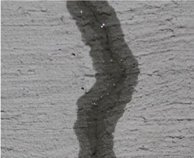
Photo 1. Insulation coating with ATLAS WODER SX on the concrete surface - water pressure from the inside. Active leak where the crack occurs in the substrate.
