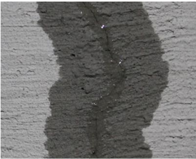
Photo 2. Gradual dampening of the insulating coating where the crack occurs.
