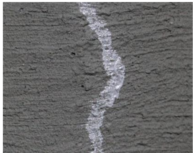
Photo 5. Slow build-up of salt crystals on the crack surface, sealing. Effect after 35 days.
