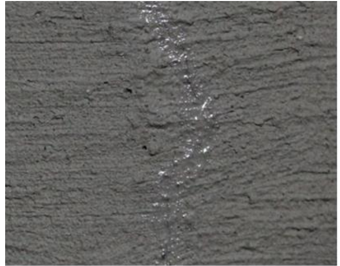
Photo 3. The crack is being gradually closed by crystallizing salts, there is still a slight water seepage. Effect after 7 days.
